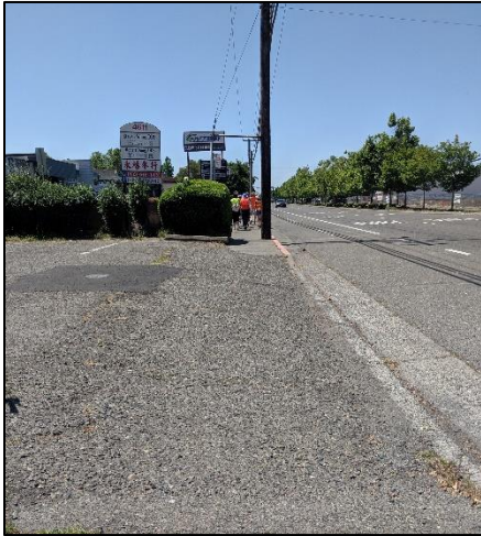
Current sidewalk and driveway conditions. Sidewalks are inconsistent and driveways are prevalent.
